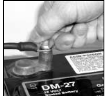
Figure 6 - Mounting temperature sensor on battery.
