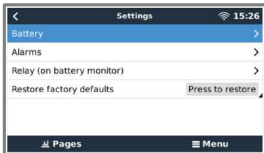
Making Lynx Shunt VE.Can settings using a GX device
